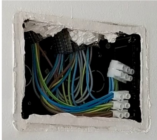
Figure 3: A type of fuse box on a Spanish home
