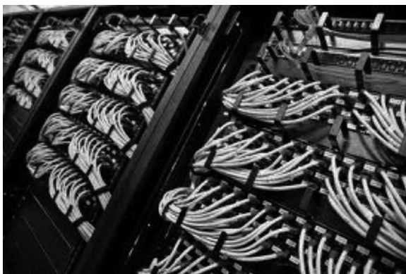
FIGURE 10.2 Networking infrastructure in data centers.
