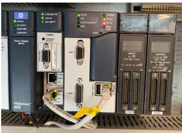
Emerson Rx3i PLC
