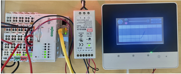
Fig. 5: PLC, Power Supply, and Microbrowser HMI A. Experimental Setup
