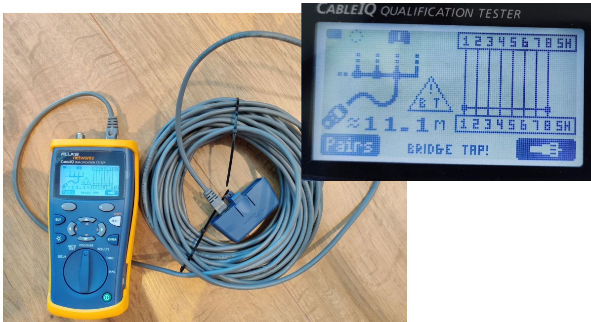
Testing a particularly faulty cable
