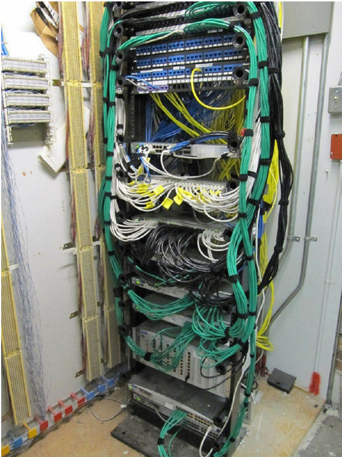
FIGURE 10.1 A typical wiring closet
