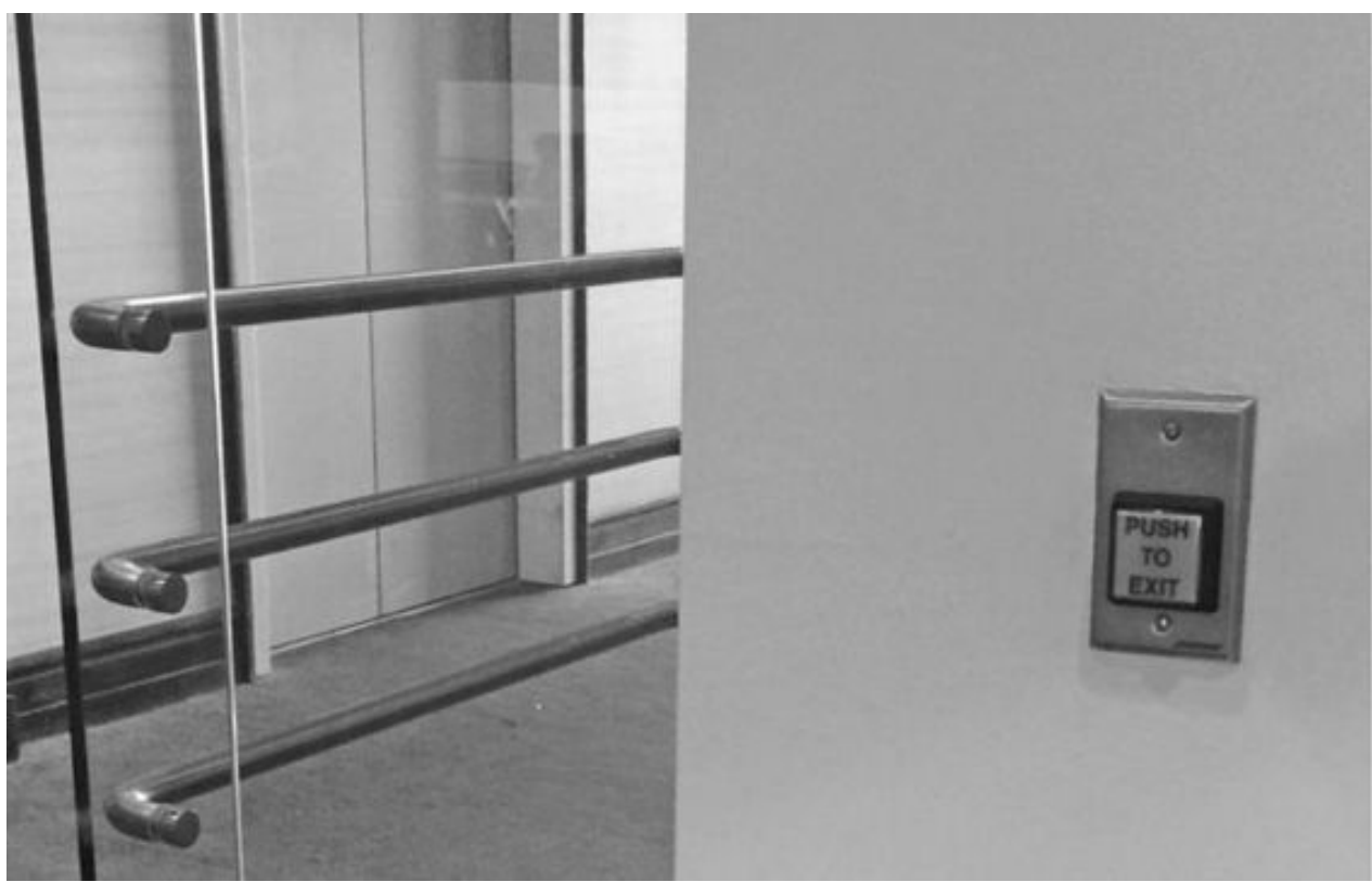
Figure 9-16 Push-button door exit
